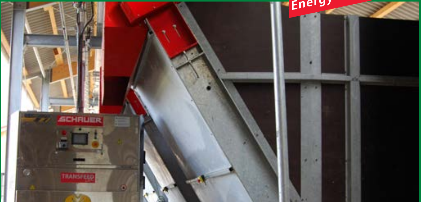
Silage pre-storage and dosing system
