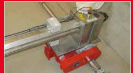
Bypass in Spotmix delivery pipe
